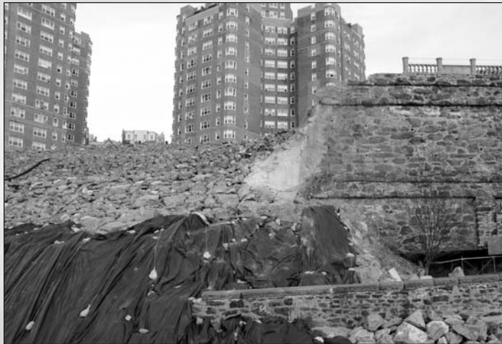
Unhappy anniversary: the collapsed wall in Washington Heights remains unrepaired nearly a year later.
