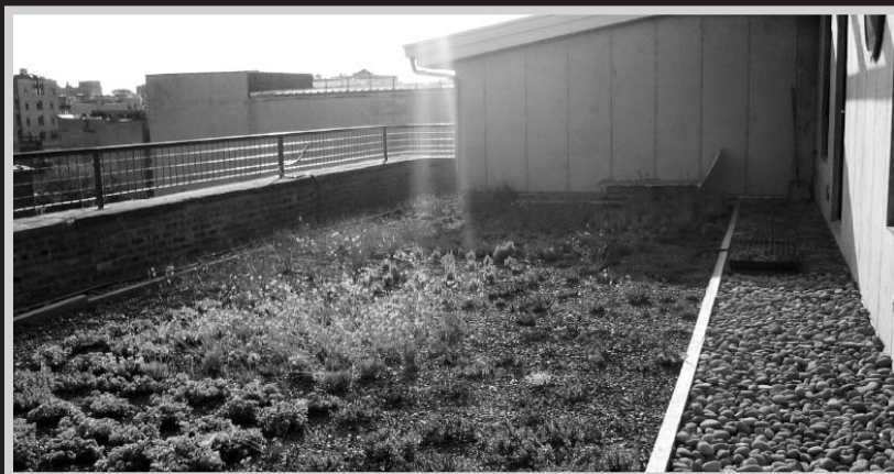
Green roofs provide insulation, reduce noise, filter air and reduce energy costs—but cost more to install than conventional rooftops.
