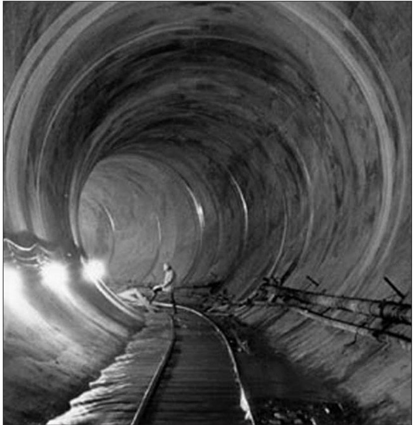
A finished section of a tunnel. [Photo source: Department of Environmental Protection]
